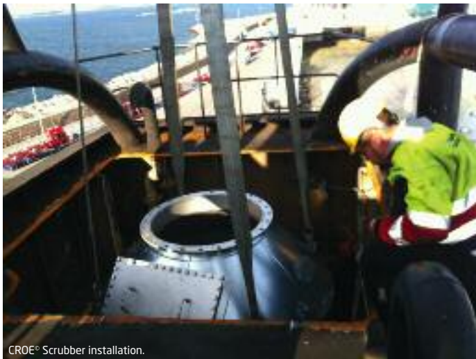
CROE® Scrubber installation.
