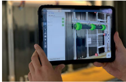
Digitised worker assistance for the installation of pipe supports Source: Sikla GmbH
